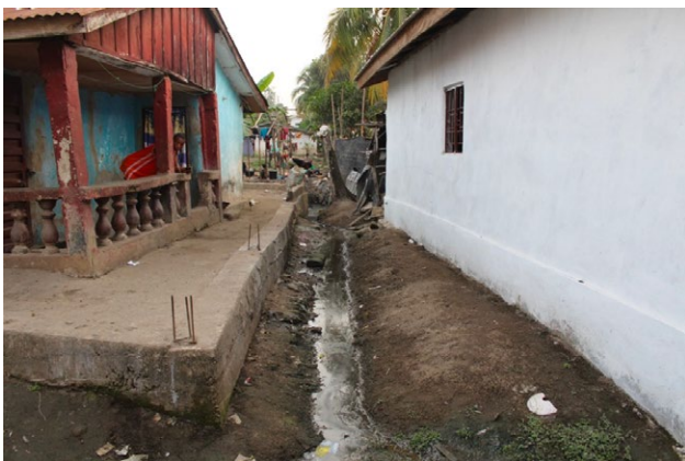
Example of poor drainage in residential areas
